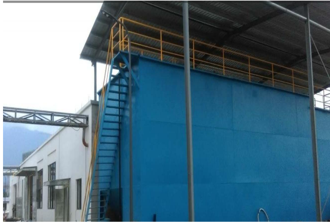
Sewage treatment equipment
